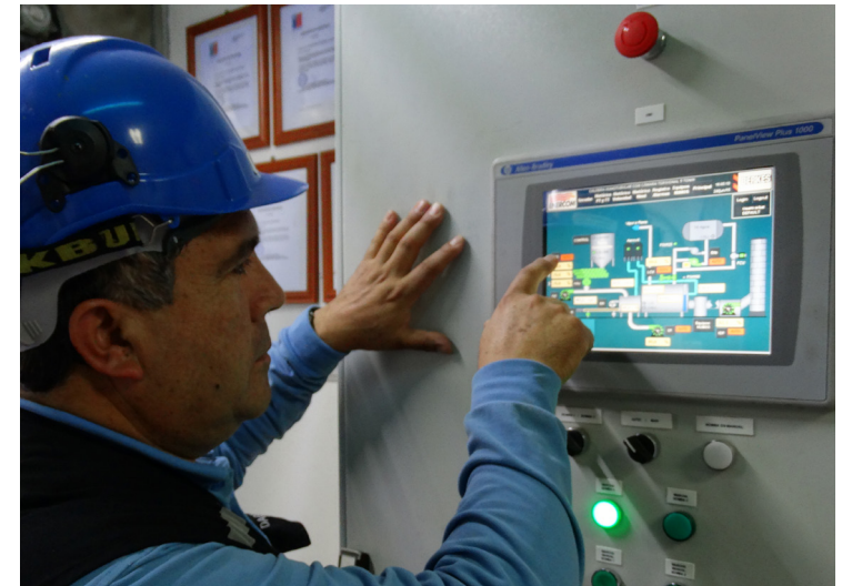
Top: The sludge drier evaporates 1,600 kilograms of water each hour, reducing water content of the sludge mixture from 68% to 10%. Bottom: Sludge boiler control panel, operated by Dagoberto Ruz. To prevent local operators’ resistance to new technologies, the company invests significant time with staff at each step of each project, researching and collecting ideas from them.
